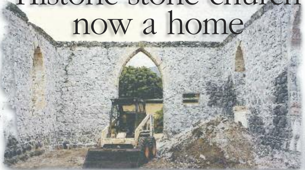
The roofless church stood for years at the end of a cul-de-sac in the quiet Waikapu neighborhood before Gary Wiest undertook the conversion to a residence in 1994.
